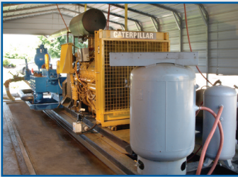
Flow Loop, Exterior
